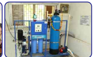
Clean Drinking Water
